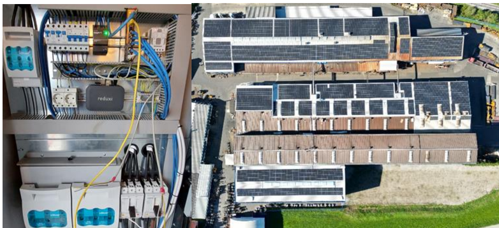
Figure 13: Example of HEMS system installation at an industrial user (left) with a 1 MW solar power plant installed (right).
